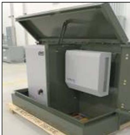
Figure 7: Power Electronics Side of International Battery CES Unit
