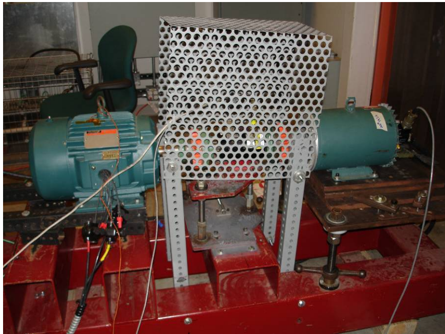
Figure 4: 5 hp Motor on Test Stand
