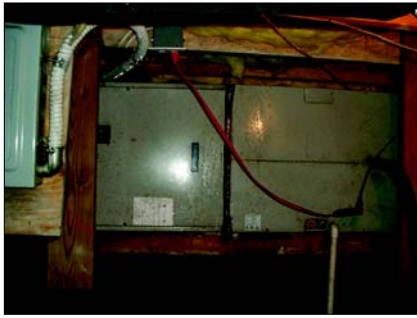
In wall-vented crawl spaces during the summer, moist crawl space air readily condenses on air conditioning ductwork. Wood framing that absorbs condensed moisture invites surface mold growth.
