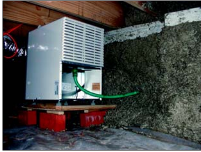
This dehumidifier is permanently installed. The green hose drains condensate directly outdoors. Note that a white termite inspection strip has been left at the top of this wall-insulated crawl space.
