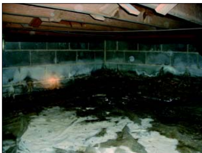
Too much water has wicked through this wall. This problem needs to be fixed before the crawl space can be closed.
