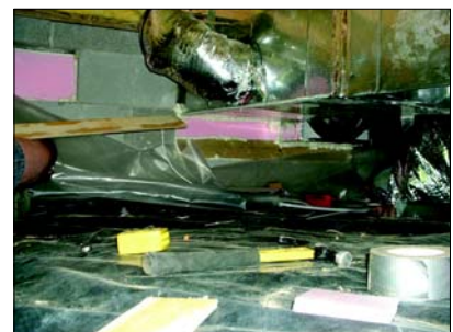
Pink rigid board insulation and expanding foam is being used to seal off the wall vent and the large opening around the ductwork that goes to the outdoor package heat pump.
