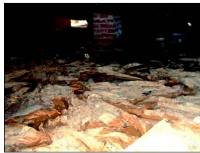
A too common sight: large puddles collect on top of the ground polyethylene in crawl spaces. Until these puddles evaporate, this crawl space will maintain high relative humidity levels that encourage mold growth.
