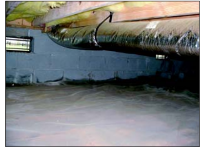
A wall vented crawl space in the study. Note that all exposed ground is fully covered with 6-mil polyethylene.
