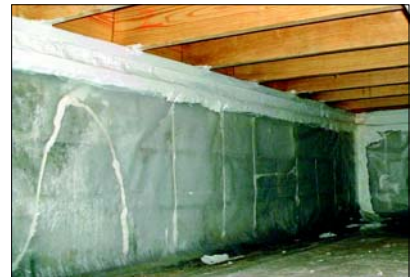
Above is a closed crawlspace in the study. The 6-mil polyethylene is brought up the wall leaving a 3-inch termite inspection strip at the top.
