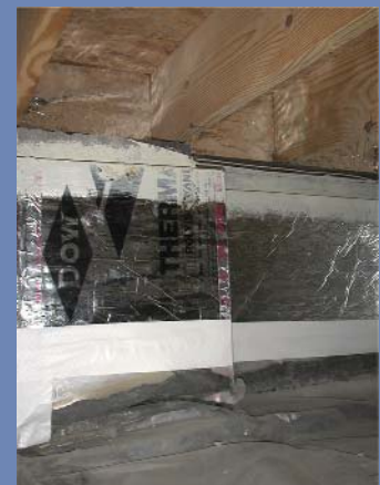
closed 2" foam wall insulation
