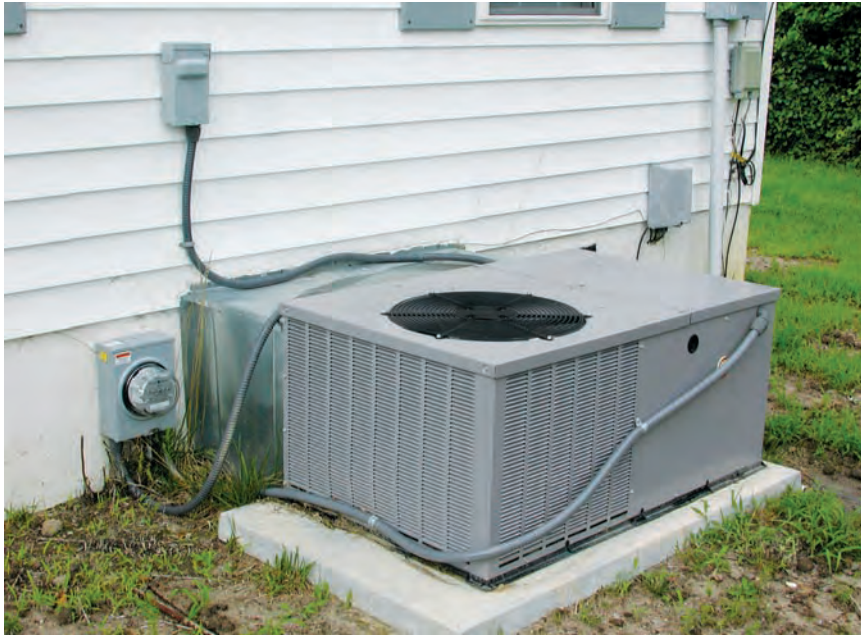
We outfitted all 12 houses with electricity submeters to record exact energy consumption by each home's package unit heat pump system.
